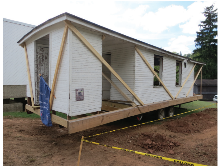
Schoonover shantyboat rests outside ORM minus its original hull. Concrete footings for a foundation will be soon be poured.
