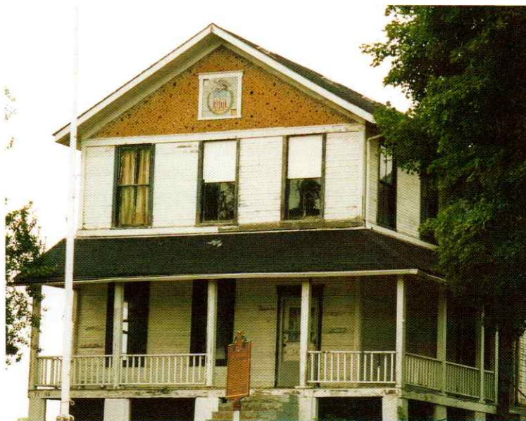
Muskingum Devol's Dam Lock House with the U.S. seal in tile at the peak of the roof dates to Corps of Engineers ownership. Judy Patsch photo
