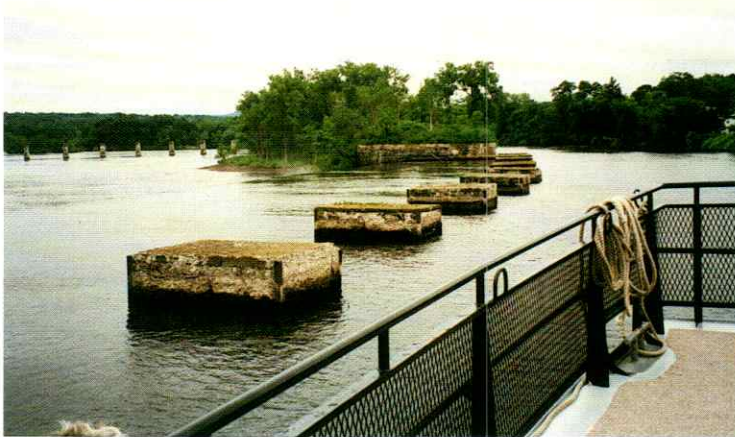
The closely spaced concrete piers keep boats safely above the crest of the dam above Lock 5, Champlain Canal. Piers in the river distant are from a railroad bridge.
