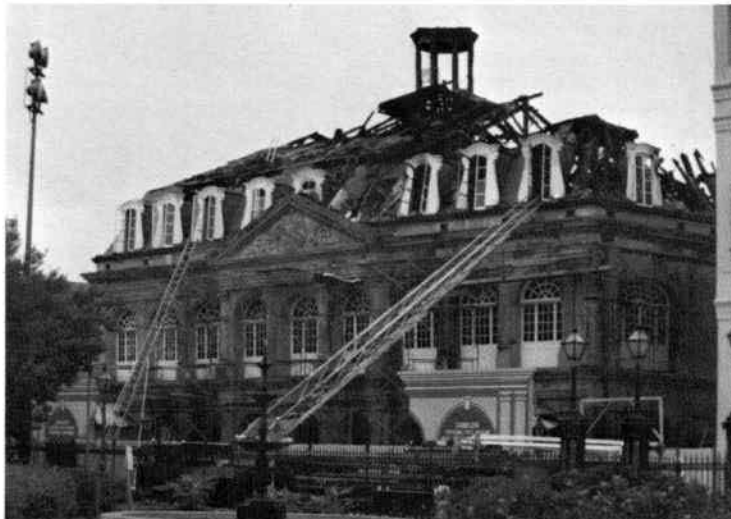
The Cabildo fire at New Orleans was really a calamity. See pages 42, 43 for details. Capt. Doc Hawley has our thanks for this view of the damage.
