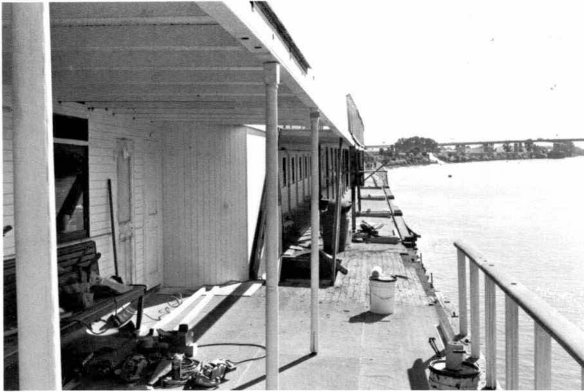
Observation Deck (where the lifeboats rested, and will again, port side looking aft. Restoration required much new decking, deck covering and railings.
