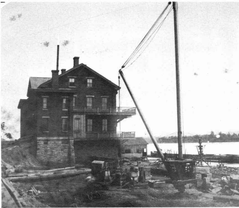
Davis Island Dam under construction, 1881. The lock house overlooks the completed lock chamber. The lock walls and lock gate recesses were constructed of cut stone and the stiff leg derrick in the foreground is set up to handle the blocks. Cut stone proved to be an expensive construction material for a project of this size and later locks were built mostly of concrete. The galleries on the lock house are an interesting feature.
